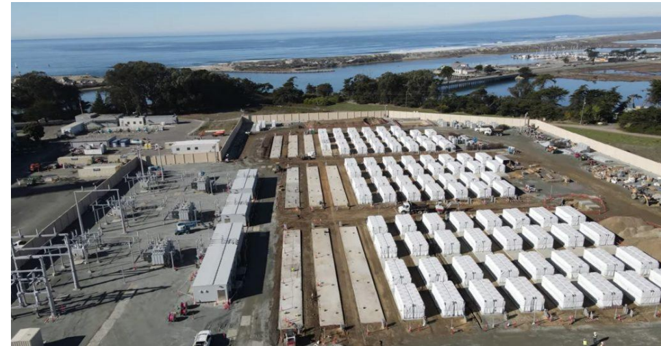
Moss Landing battery storage
